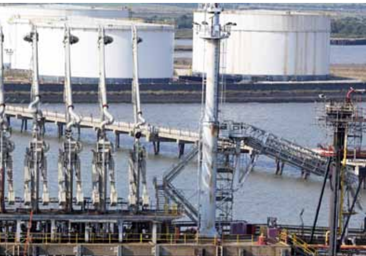
Tank terminal with loading arms
