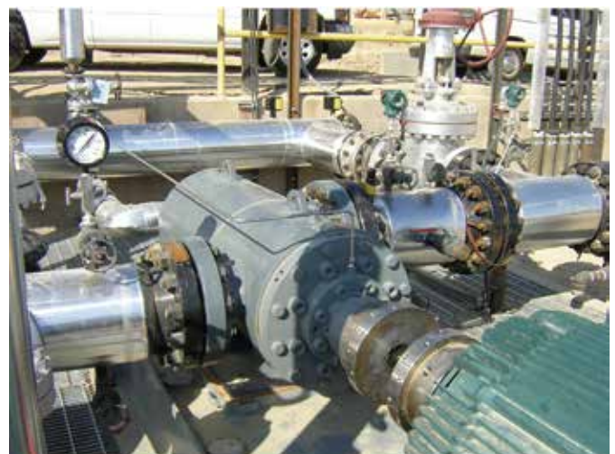
crude transfer pump
