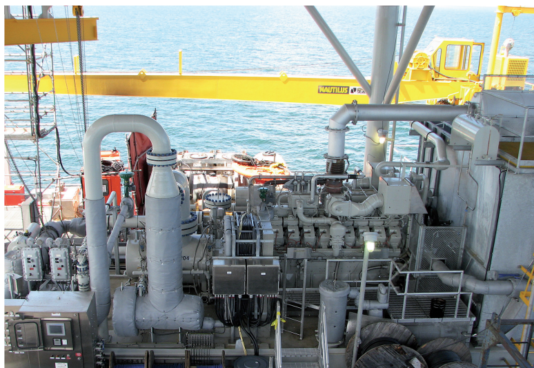
Fig. 2: Multiphase booster pump on a wellhead platform
