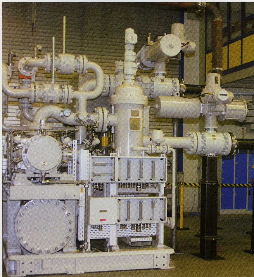
Fig. 2 Multiphase Pump Skid on the Multiphase Pump Test Bed
