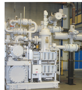
Multiphase pump skid on the multiphase pump test bed
