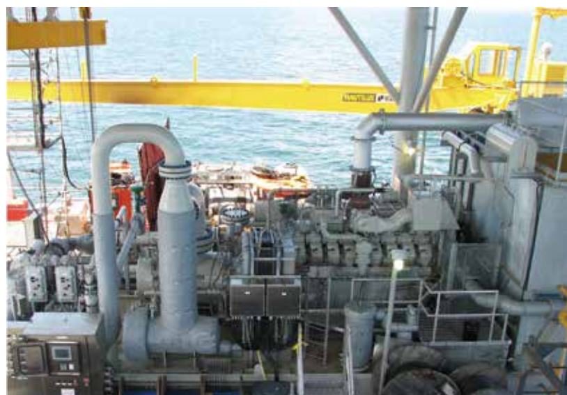
Multiphase booster pump on a wellhead platform
