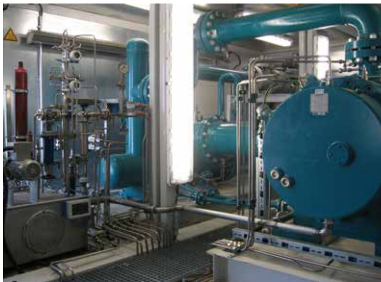
Leistritz multiphase pump system installed in a container
