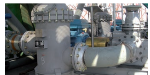
4 Electric Dehydrator Feed Pump L4
