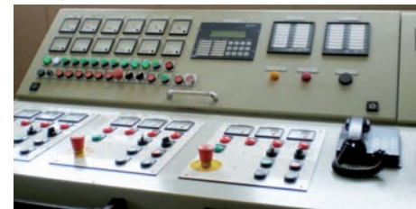
Control apparatus mounted in Cargo room
