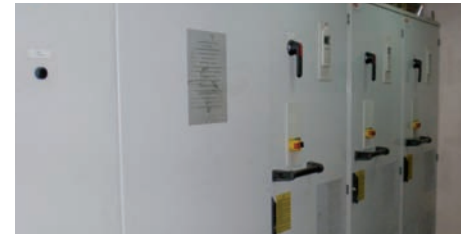
Frequency Converter Cabinet
