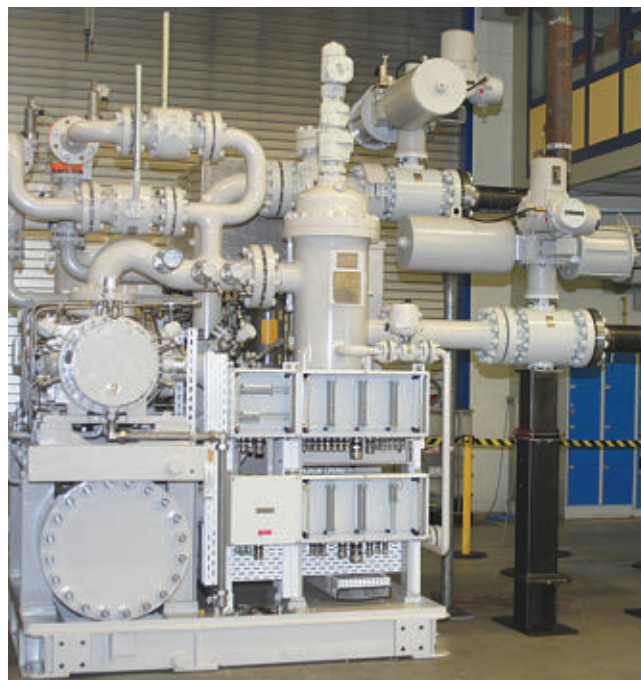
■ The wellhead platform includes this multiphase pump skid.
