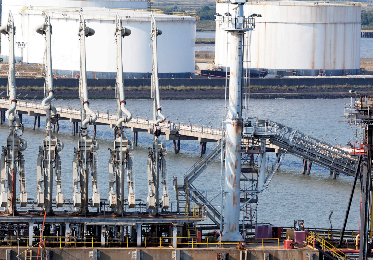
Tank terminal with loading arms: Innovative and more flexible pumping systems can make big contributions to a flexible, smooth and cost-efficient operation of oil and tank farms.
