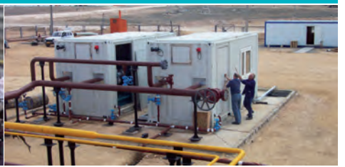
Containerized Leistritz Multiphase Pump in a Permafrost Area in Kazakhstan
