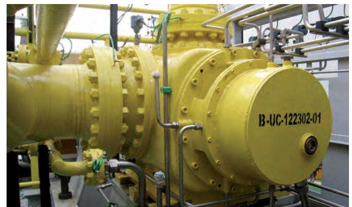
Leistritz Multiphase Pump System on an Offshore Platform in Brazil
