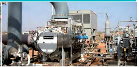
Leistritz Multiphase Pump Installation on an Oil Field in Central Africa
