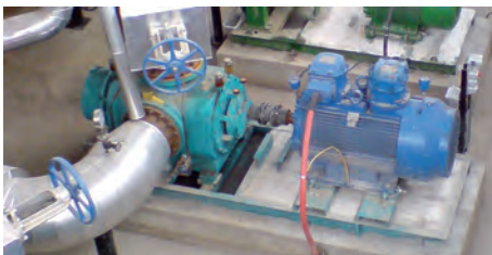
4 Seal Oil Pump L3HF
