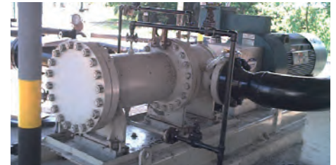
3 Crude Booster Pump L3HG
