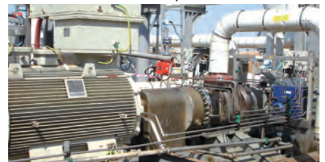
2 Pipeline Start-Up Pump L4HK
