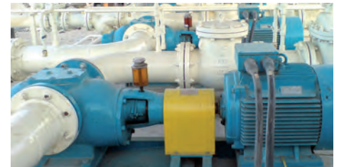
2 Crude Unloading Pump L2NG
