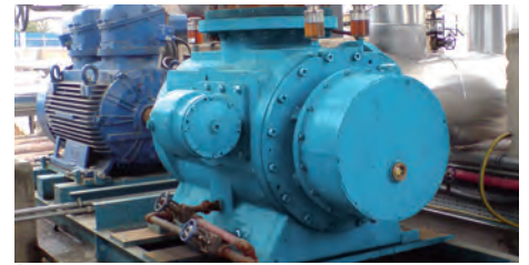
2 Circulation Pump L4MG
