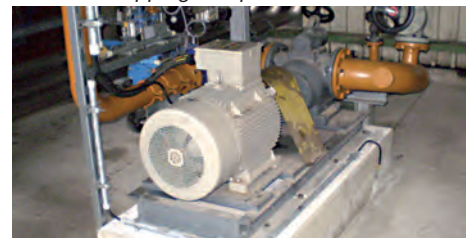
5 Tank Cleaning Pump L4NG
