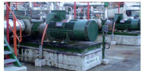
2 Crude Charging Pump L4NG
