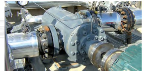
4 Crude Transfer Pump L3MG
