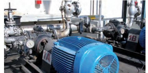
4 Slops & Drains Oil Pumps L2NG
