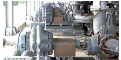
3 Crude Transfer Pumps L2NG
