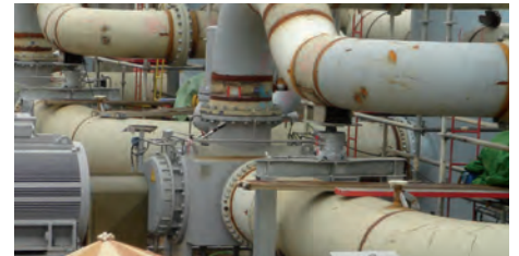
3 Loading and Transfer Pump L4NG
