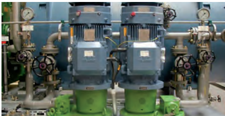
2 Auxiliary Lube Oil Pump L3MF
