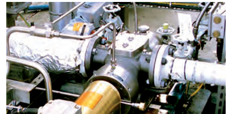
2 Chemicals Handling Pump L4NG
