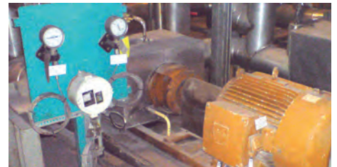
4 Crude Stripping Pump L4NG
