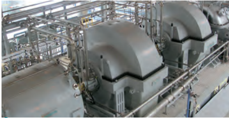
1 Compressor Lube and Seal Oil Pump L3
