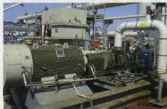
Pipeline start-up pump in Africa
