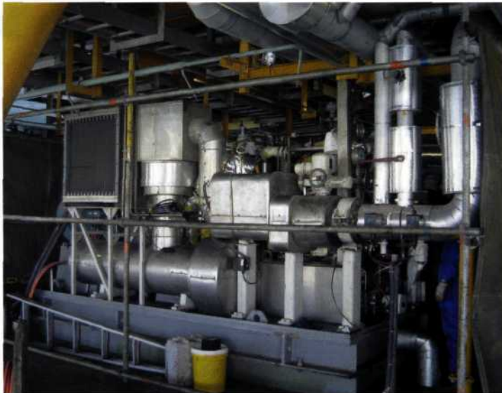
Electric motor driven multiphase pump with insulation on an offshore platform in China (photo: Leistritz Pumpen GmbH)
