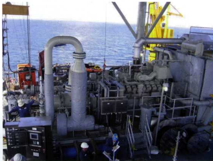
Multiphase pump package with gas engine and liquid management system on an offshore platform in the Gulf of Mexico (photo: Leistritz Pumpen GmbH)
