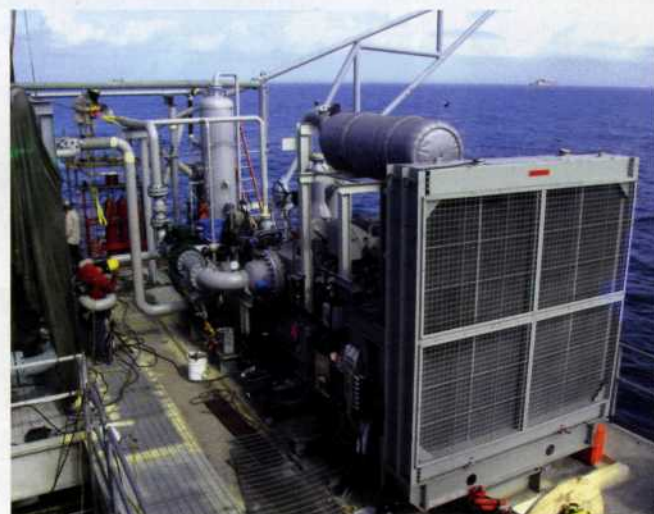
Gas engine driven multiphase pump on an off shore platform in the Gulf of Mexico Mexico (photo: Leistriz Pumpen GmbH)
