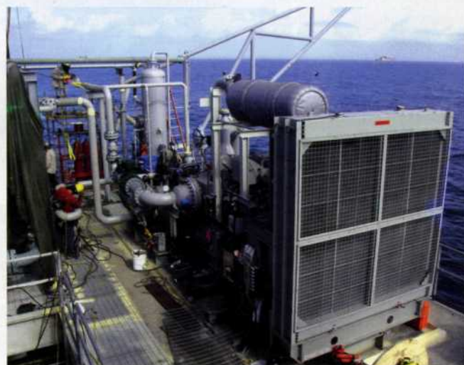
Gas engine driven multiphase pump on an off shore platform in the Gulf of Mexico Mexico (photo: Leistriz Pumpen GmbH)
