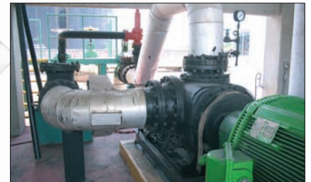
1 FO Unloading Pump L4NG
