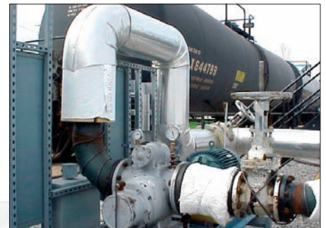
1 FO Unloading Pump L2NG
