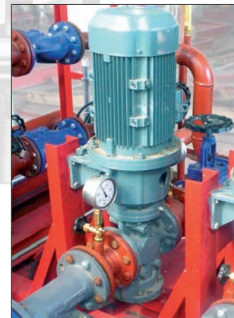
3 4 10 11 FO/DO Transfer and Separator Supply Pump
