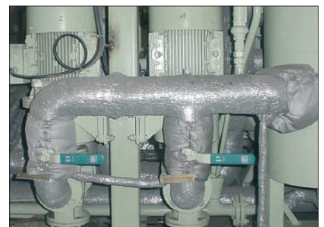
5 6 FO Feeder and Booster Pump L3NG
