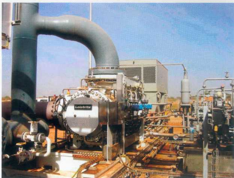
Multiphase Pump application with external re-circulation system in Chad
