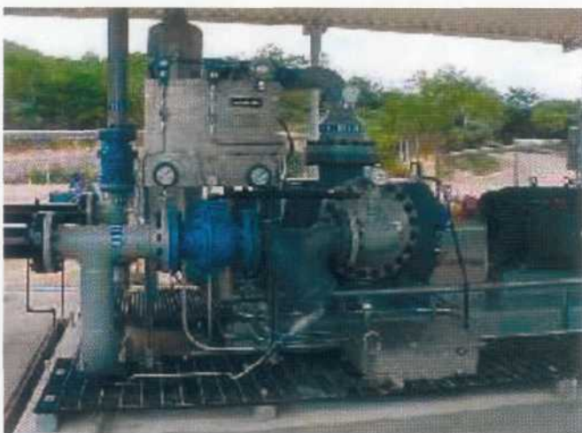
Multiphase Pump installed on a remote field in Colombia
