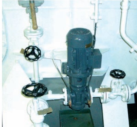
2 3 6 LO Separator Supply, Cylinder Oil Transfer and Crosshead Lube Oil Pump L3NG
