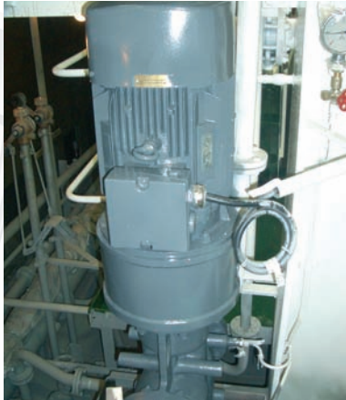
1 5 LO Transfer and Pre Lube Oil Pump L3NG
