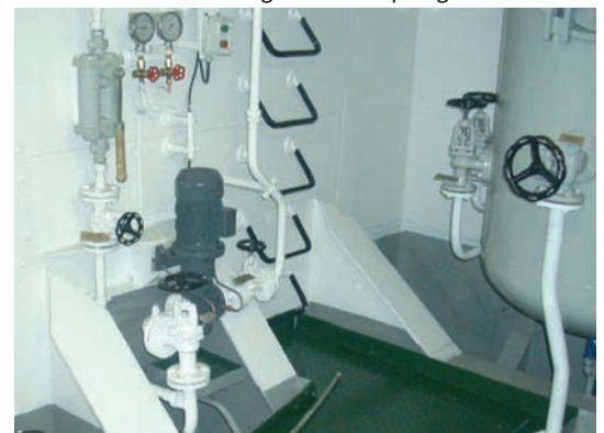
5 7 Diesel Oil Booster and Boiler Supply Pump L3NG
