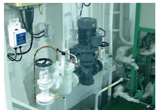
6 8 9 Fuel Oil, Diesel Oil Boiler and Separator Supply Pump L3NG
