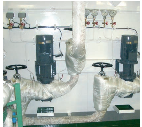
3 4 Fuel Oil Feeder and Booster Pump L3NG with Magnetic Coupling
