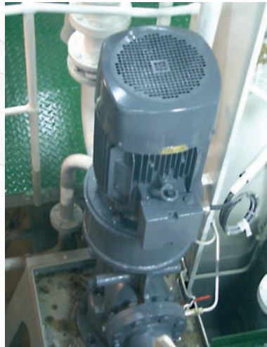
1 2 Fuel Oil and Diesel Oil Transfer Pump L3NG
