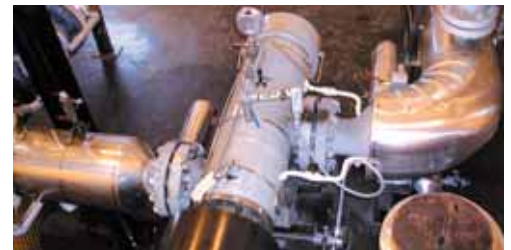
3 Leistritz HFO Booster Pump L3MG
