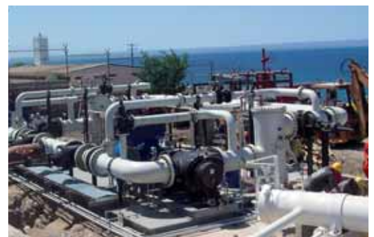
Heavy Fuel Oil Unloading Pump in Mexico
