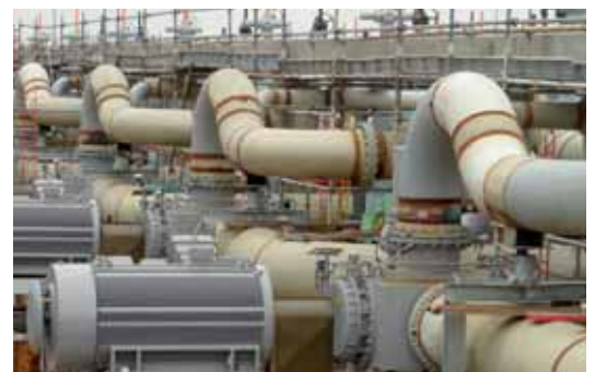
Ship Loading Pumps in Singapore
